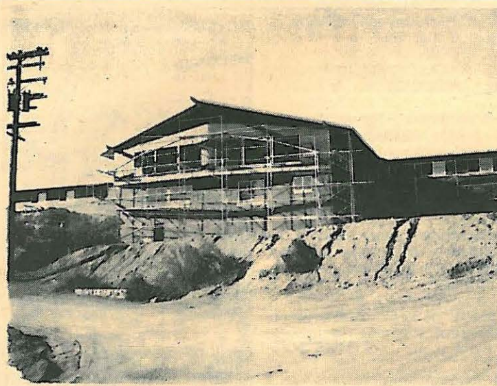
Work continues on the beautiful new addition to the Alpine Convalescent Center.
